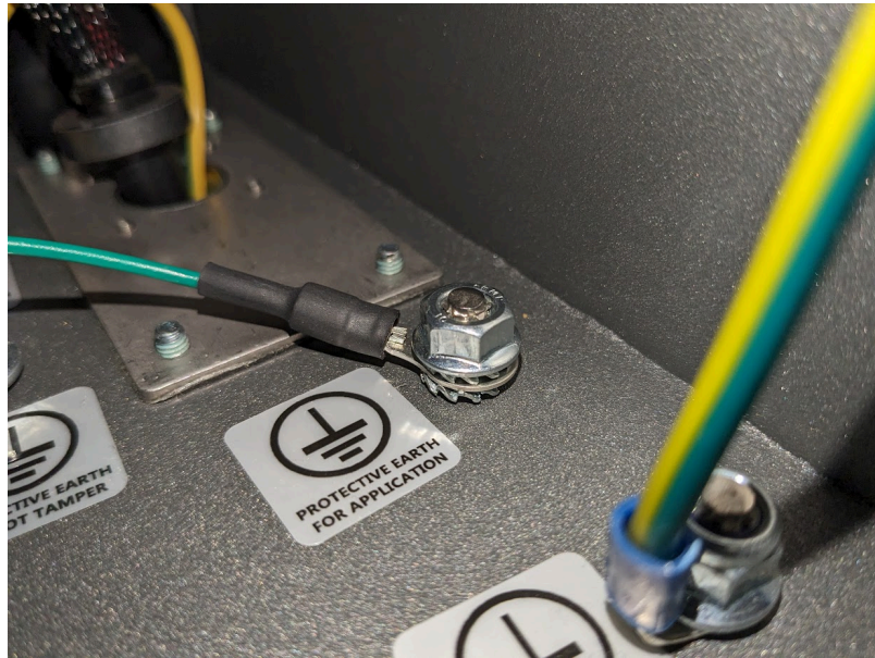
Fig. 3-20: Example of Ground Connection in Robot Control Box
